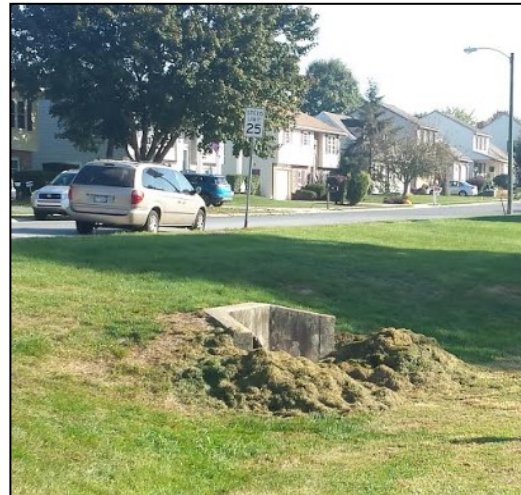
Illicit dumping of grass clippings into a detention basin outlet.
